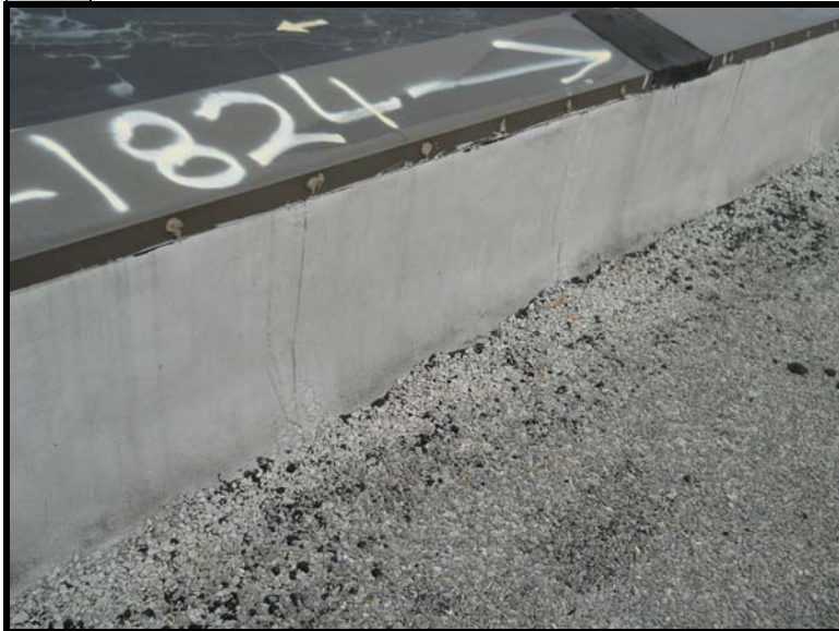
3 The silver paint located on the front parapet of most of the Stores tested positive for asbestos (2% chrysotile).
