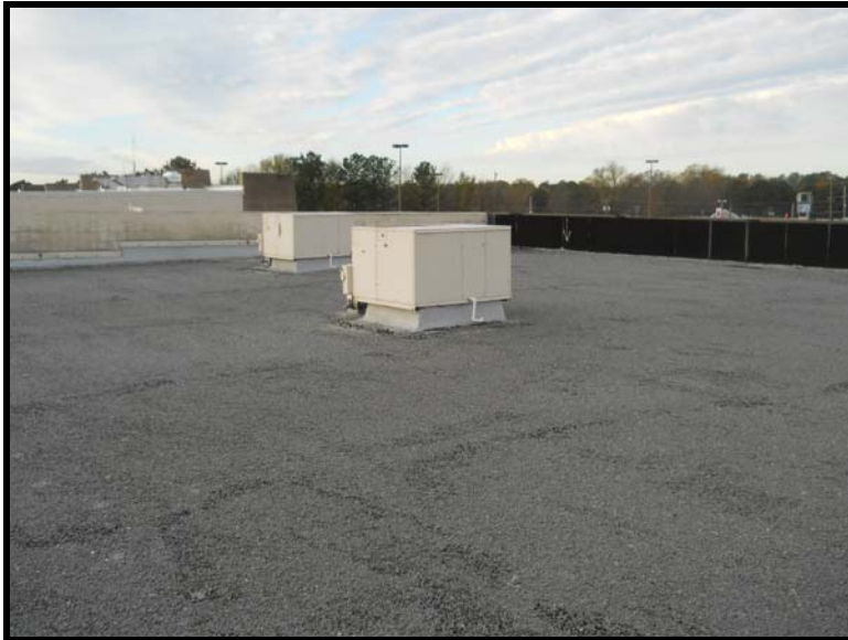
5 The roof over Stores 1848 and 1852. The black flashing on the front parapet of these stores did not test positive for asbestos.
