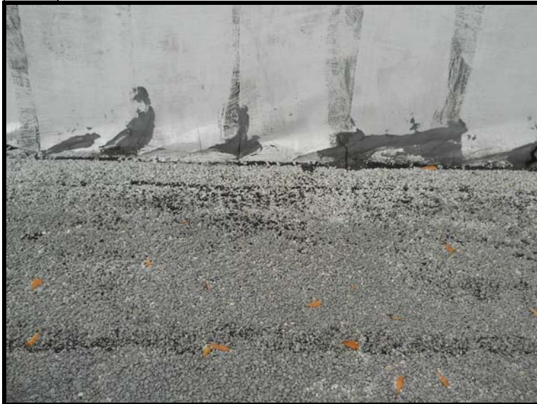
7 The roof and parapet at the front of Store 1872. The silver paint located on the front parapet tested positive for asbestos (2% chrysotile).
