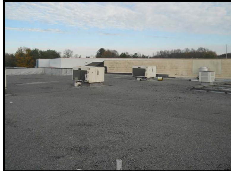
4 The roof over Stores 1840 and 1844. The silver paint located at the base of the A/C units tested positive for asbestos (2% chrysotile).
