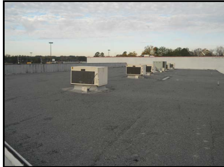
6 The roofing system over Stores 1856 through 1872. The silver paint located on the front parapet and under the A/C units tested positive for asbestos (2% chrysotile).
